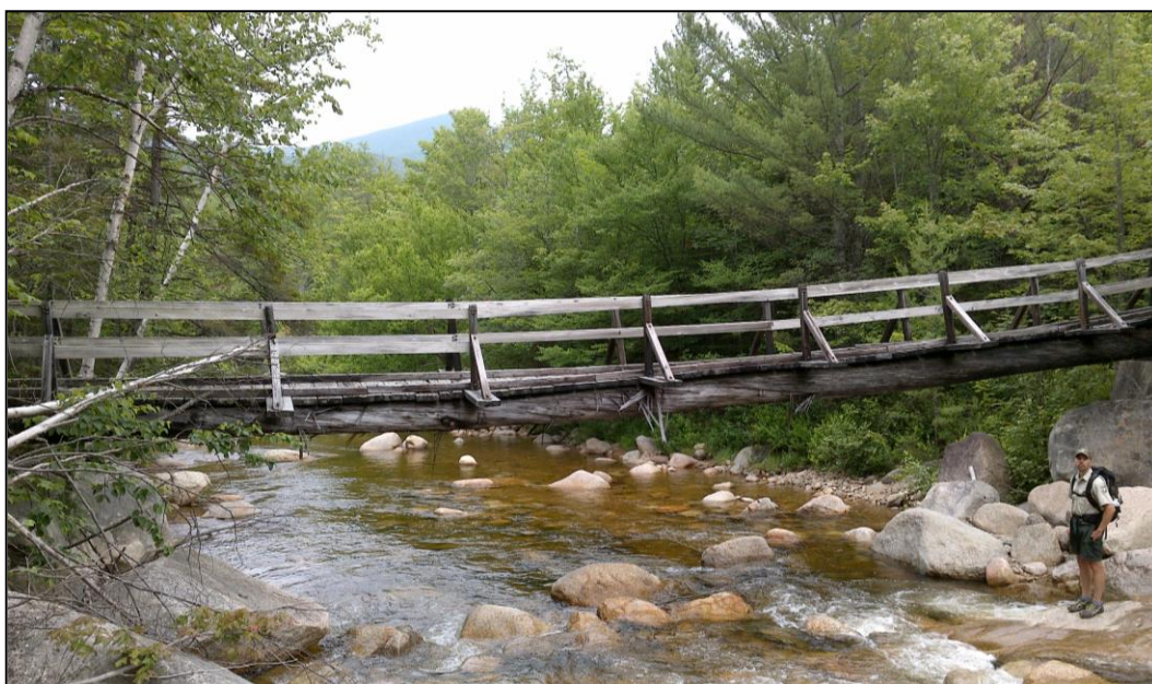
Figure 4. Time and storm damage have resulted in delamination and cracking of the stringers and sagging of the Thoreau Falls Bridge structure. For safety reasons, the bridge has a one-person at a time weight limit.
