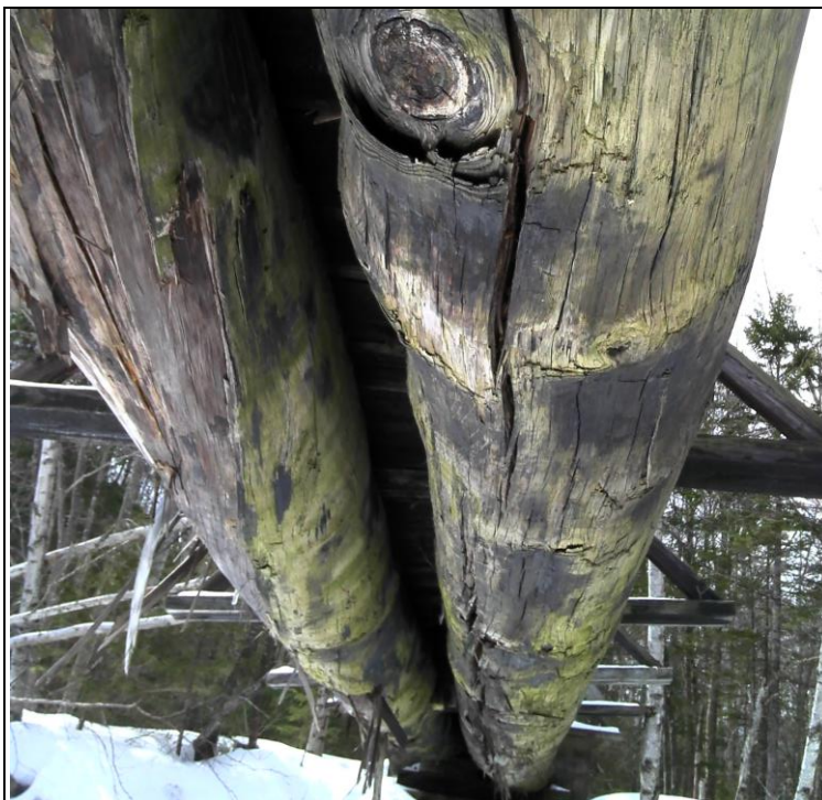
Figure 7. Cracks and delamination of stringers.
